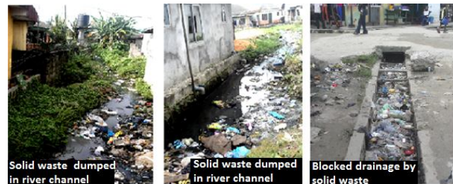
Fig. 7: Solid Wastes Dumped into Water Channels and Drainage that clogged drainages that enhance severe Flooding in the city
